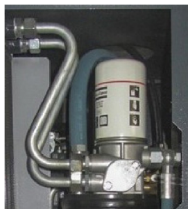
Figure 14: Safety valve on the compressor - Detail
