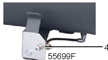
Figure 40: Condensate drain valve on air receiver
